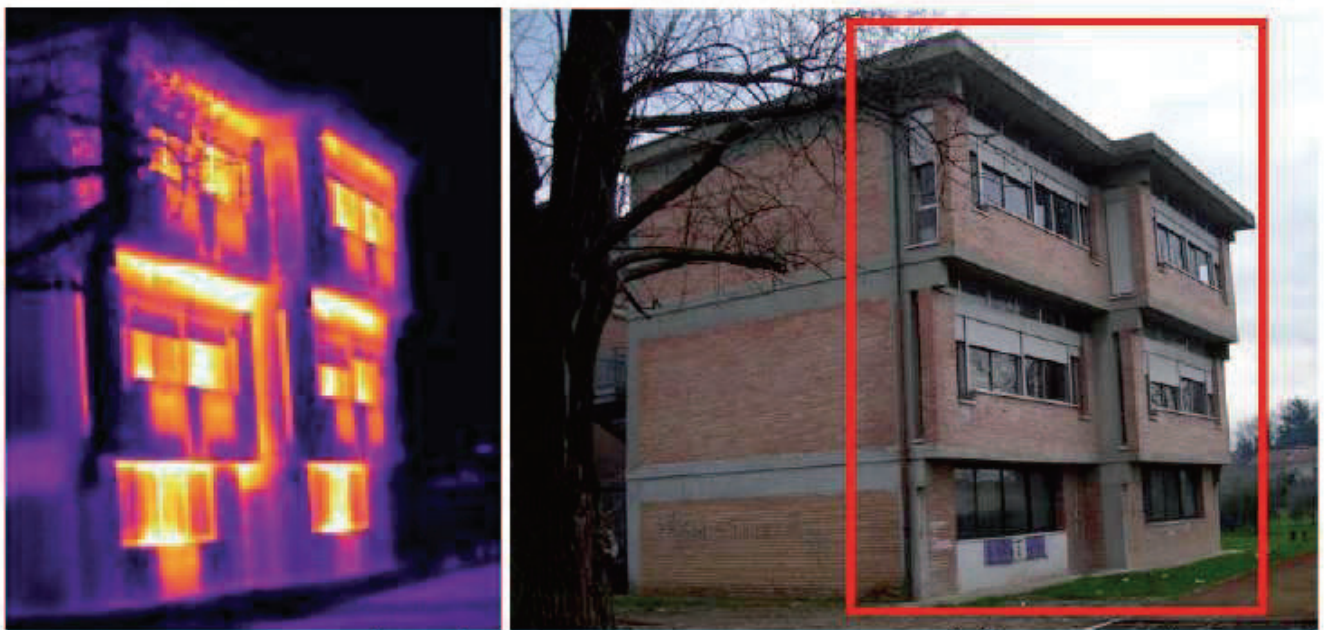
Figure 1: Thermography has been a fundamental instrument in the diagnosis phase: heat losses can be localized easily
