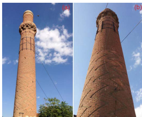
Figure 1. Photos of Minaret: (a) General view; (b); Steel cables and clamped part of minaret.
