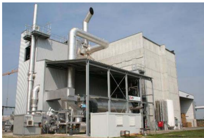
Figure 10: SP rotary pilot plant in Dürnröhr, Austria [34].
