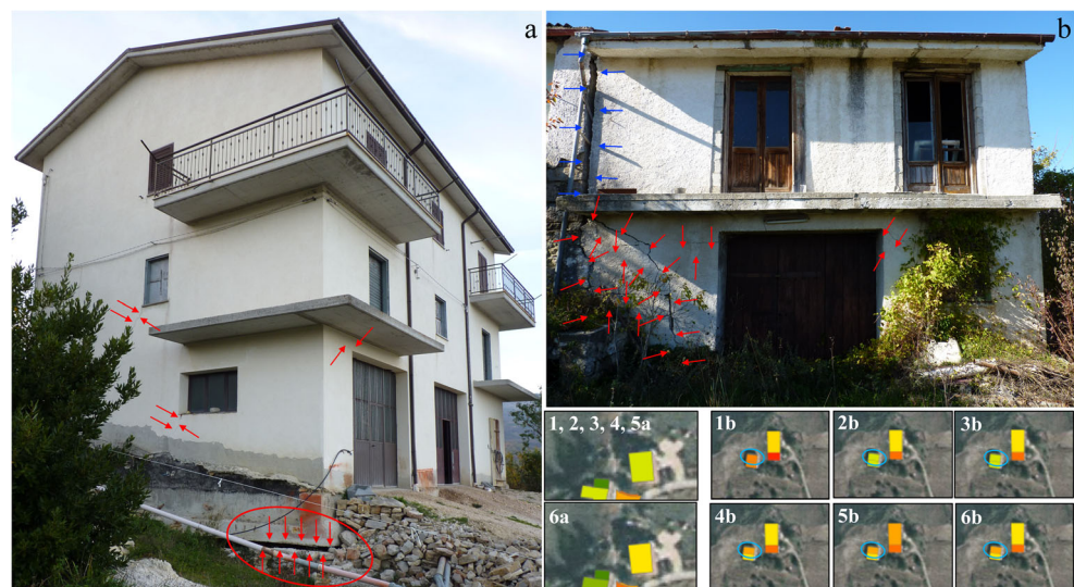
Fig. 12 Damage assessment for two buildings located in the study area by means of different approaches: a) three-level concrete structure located close to the landslide crown; b) two-level masonry building positioned on the left flank of the landslide. Both edifices were classified according to the (1) Burland et al. (1977), (2) Alexander (1986), (3) Chiocchio et al. (1997), (4) Cooper (2008), (5) Baggio et al. (2009), and (6) Del Soldato et al. (2017) approaches. Damage are highlighted by red arrows, and open joints between the nearby structures are shown in blue
