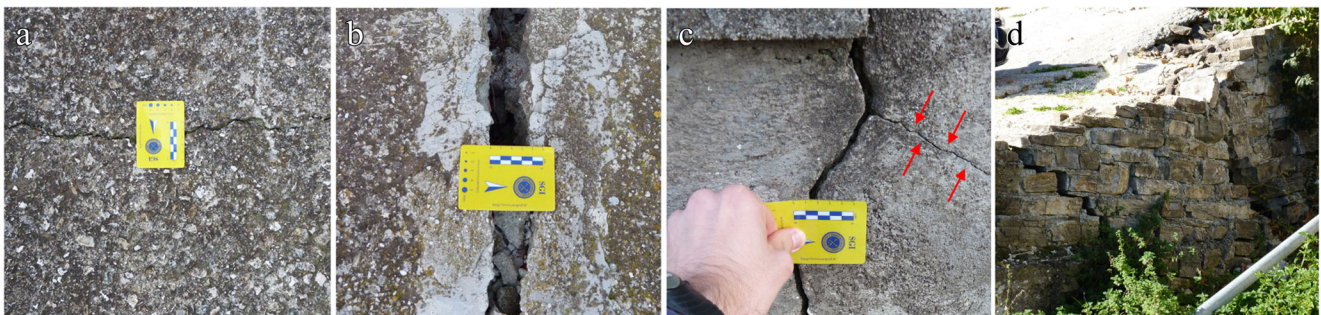
Fig. 8 Damage recognized on concrete slabs and walls. a) Hairline crack in pavement; b) open rupture in a slab; c) hairline (red arrows) and open fractures in a concrete wall; d) damage to a masonry wall
