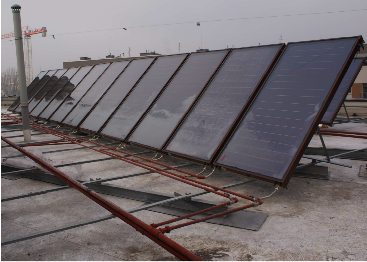
Fig. 6.6 Solar collector row (one of three) on the roof in Wrocław 2
