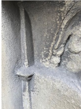
Figure 4.1 Black deposition on stone surface.
