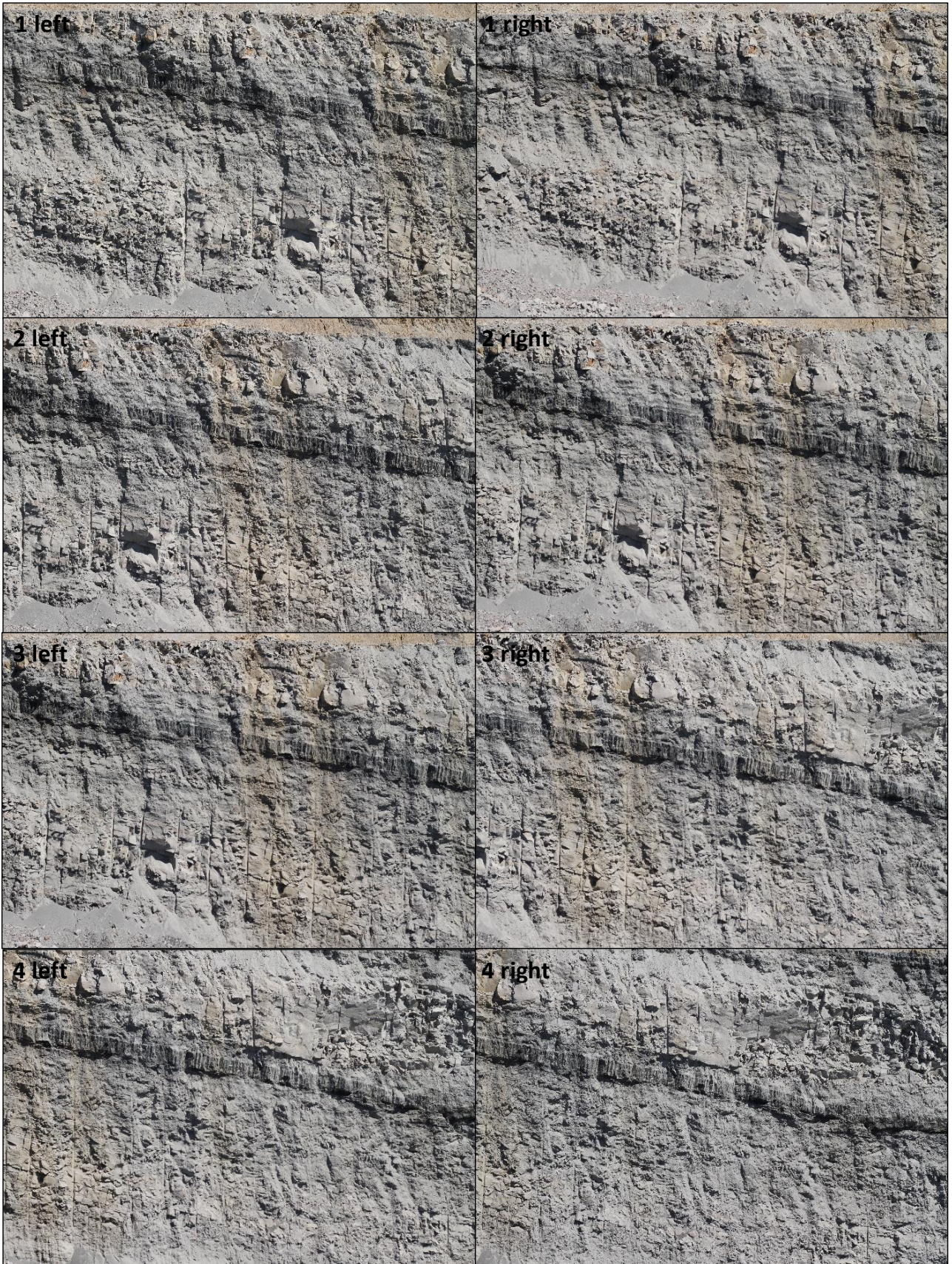
Figure 87 - Images of case study 2 highwall. The numbers indicate the order of the stereo pairs of Figure 86, from left to right
