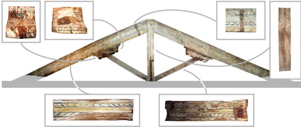
Fig. 1. Decorated truss n. 1. Picture rearranged by mosaic composition. The sign of king-post stirrup (+) in its original position, rotated and centred onto the tie-beam (nowadays under the floor)
