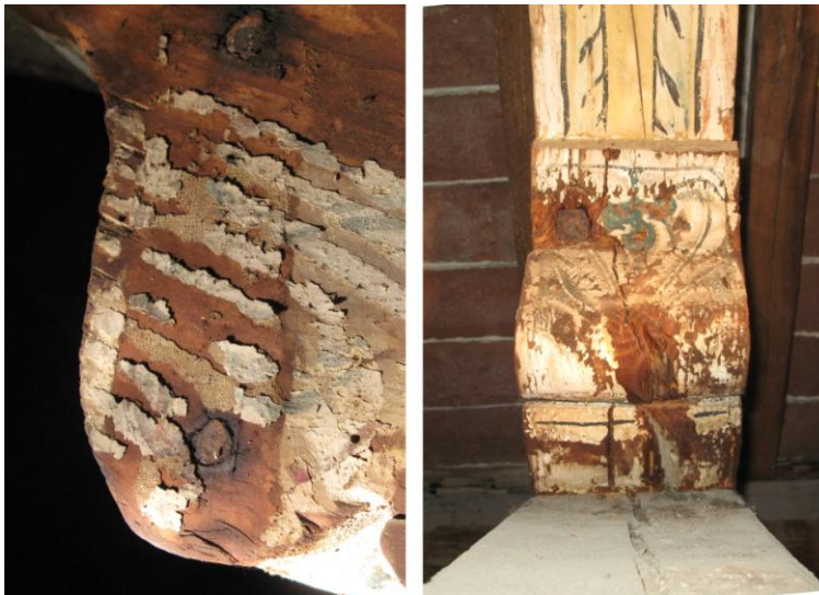
Fig. 2. Example of fabric on structural timber. Left: strip of fabric, residual on earlywood, to cover two nails. Right: end-grain of a cantilever with fabric (still present, with gaps) to upholster nails and a shrinkage fissure
