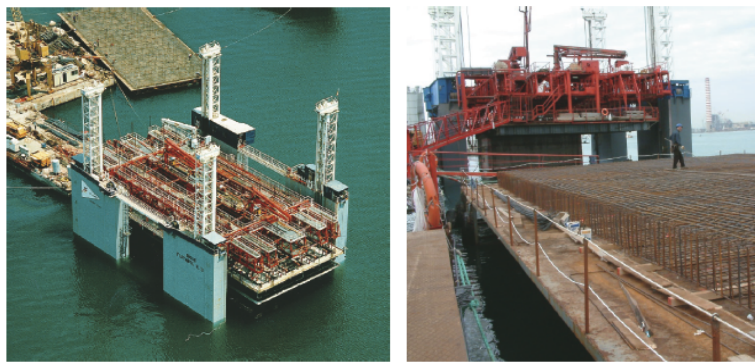
Fig. 3.4 - a) (on the left) Concrete caissons pier of Enel Thermal Power Plant at Torrevaldaliga (RM), b) (on the right) the Spanish company DRACE.
