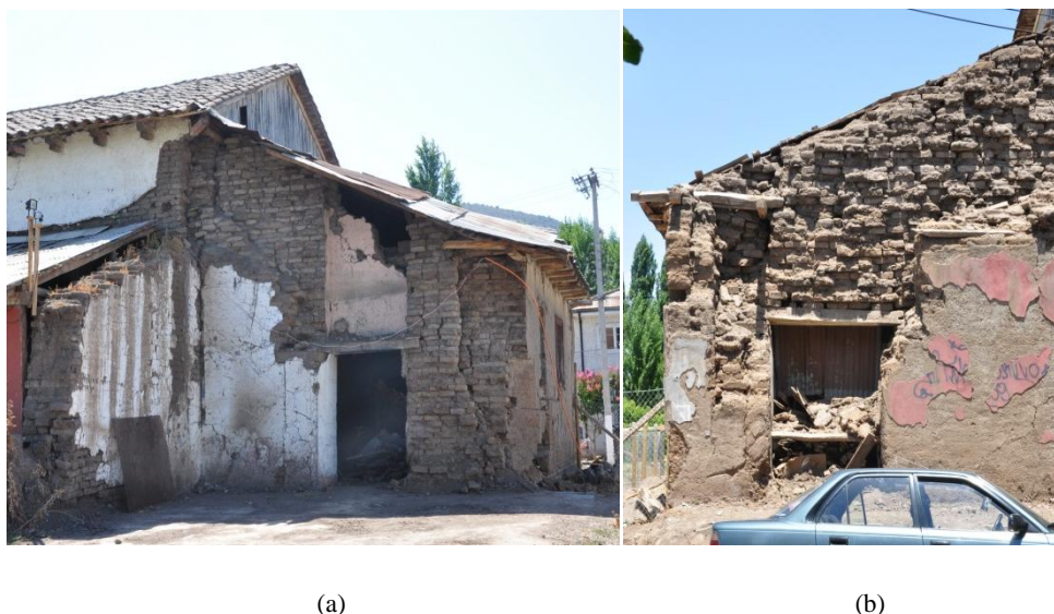
Figure 5.1.10 - Local collapses of Sacristy (Surtierra, 2011).
