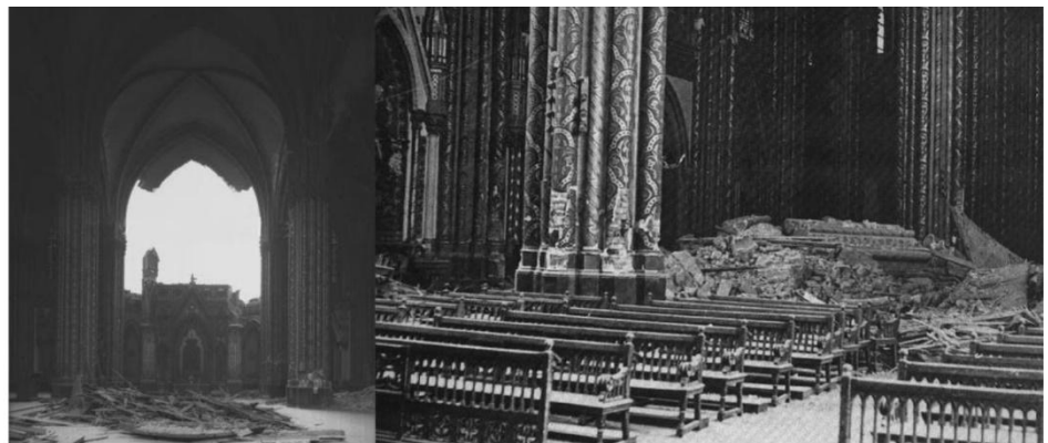
Figure 5.3.3 - Photo (a) west transept wall, and (b) two central nave columns, collapsed after the 1985 earthquake (Ministry of Public Works).
