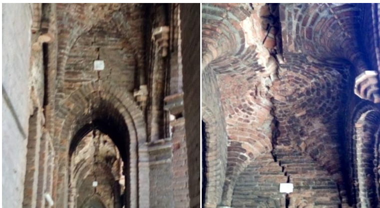
Figure 6.2 – Deep cracks in the transverse arches of external gallery of Basilica del Salvador.
