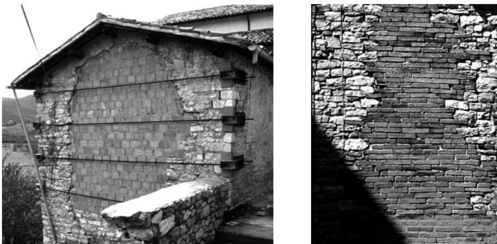
Figure 6.12 - Masonry replacement intervention. The repairs are ineffective due to the lack of compatibility between the masonry portions (Frumento et al., 2006).
