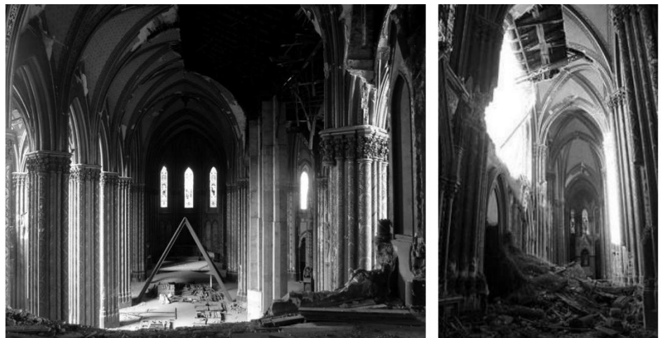
Figure 5.3.4 - Photo (a) and (b): worrying crack pattern and local failures of east side aisle wall, central arch of narthex, arcades of the external gallery and columns of the central nave. (Ministry of Public Works).
