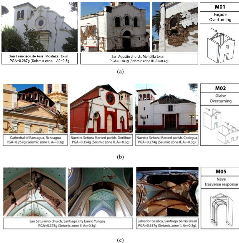
Figure 4.5 - (a) Out-of-plane mechanisms of the façade due to poor connections at the corners: in the San Francisco de Mostazal the simple overturning involved the central part of façade, and in the San Agustín church the complete façade; (b) gable overturning effect of inadequate connection between roof structure and masonry wall of the upper part of façade on Cathedral of Rancagua, Doñihue's parish, and Codegua's church; and (c) observed collapses on the haunch of the transverse arches of side aisles
