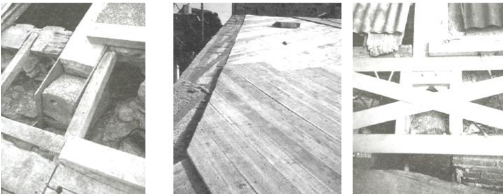
Figure 6.4 - Steel ring beam: a) connection between the wood roof element and the walls; b,c) partial strengthening of the plywood panel diaphragm and its connection with the steel ring beams (Regione Marche 2000). (Frumento et al., 2006).
