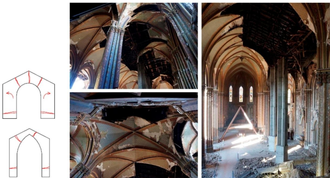
Figure 5.3.11 -Collapses of the transverse arches and arches of the longitudinal west wall.
