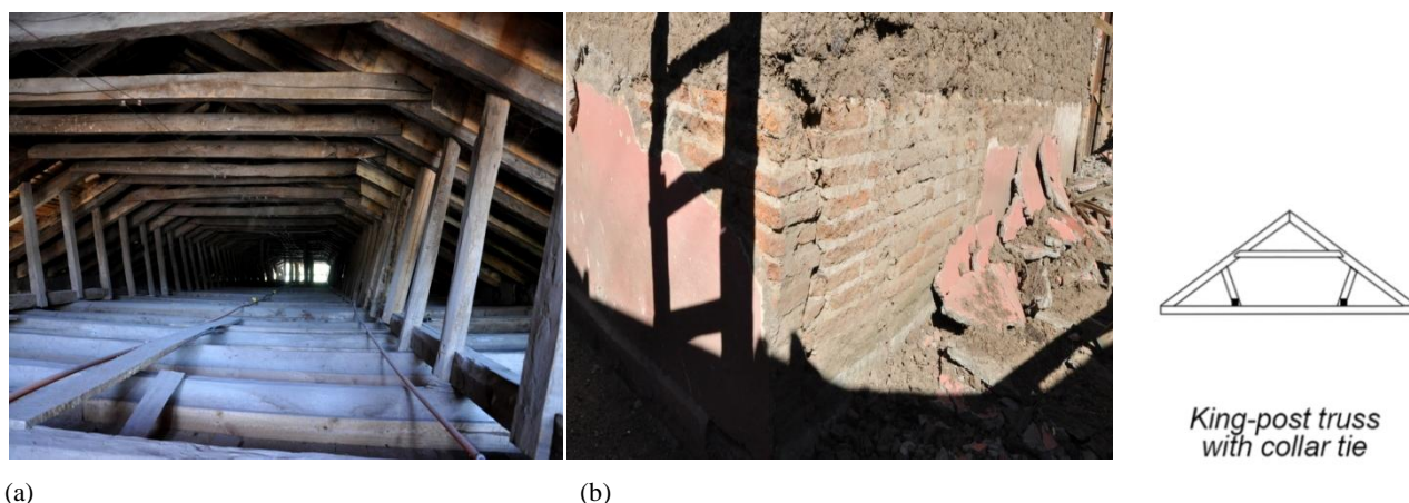
Figure 5.1.5 – Roof system of (a) traditional timber king-post trusses with collar tie, and brick basement of foundation visible of the external lateral façade (Surtierra, 2011).
