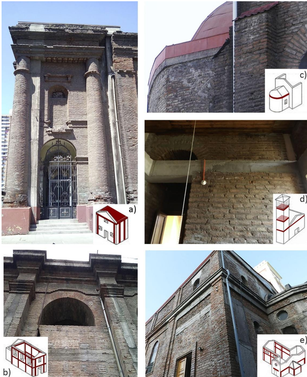
Figure 2.2 - Reinforced Concrete (RC) interventions in some churches in Santiago: a) RC slab in the narthex of San Isidro Labrador church; (c) and (d) RC ring-beam in the apse and bell tower of San Pedro's church; and (e) RC tie rods in Santa Sofia's Parish and (b) Dominicanana church.
