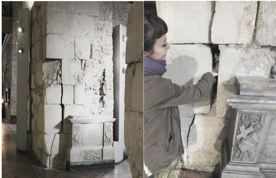
Figure 6.19 - Worrying deep vertical crack in arch piers of central nave pillar axis F.
