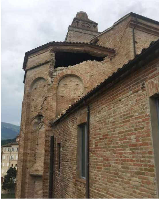
Fig. 1 Amandola, province of Fermo: the apse of San Francesco church damaged by the recent earthquake. (July 2018)
