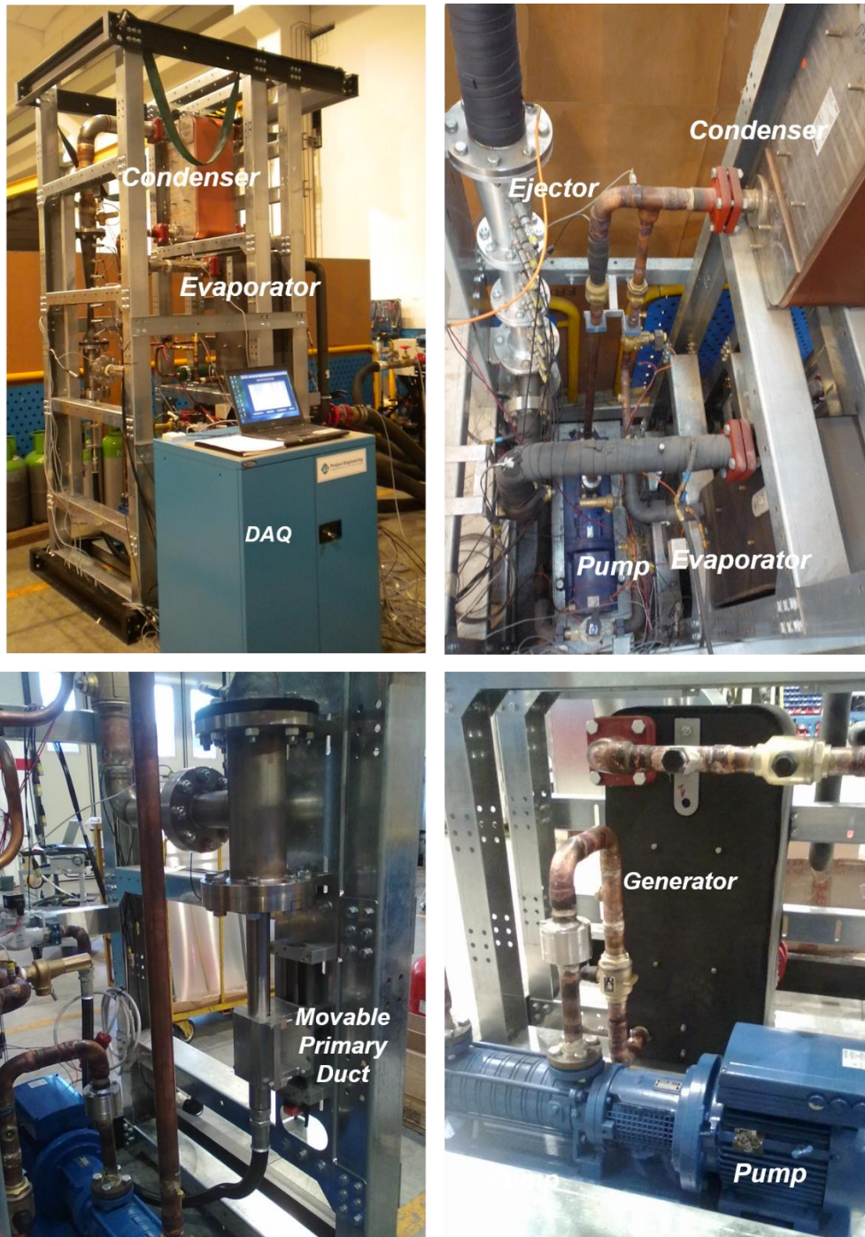
Fig. 6.3. Pictures of the chiller
