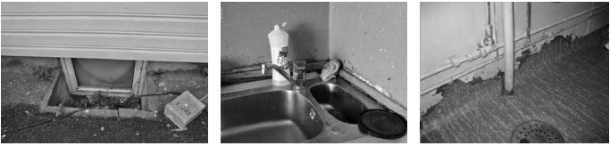
Fig. 2. Examples of low standard and moisture problems in decentralized reception centres. Left: Sleeping room window with insufficient daylight conditions (photo: K. Denizou). Middle and right: Worn down surfaces and moisture in kitchen and bathroom (photos: R.Ø. Thorshaug).
