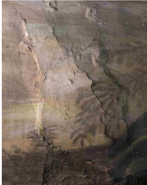
Figure 1.2 Wall cracking of Villa Farnesina caused by traffic vibration (Feiden 2007)
