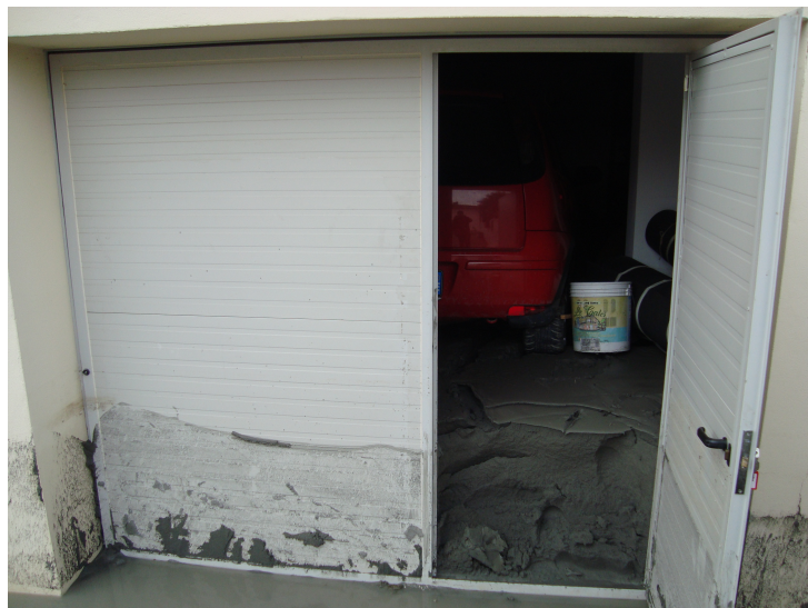
Figure 2.2: Lifted up pavement of a box auto after the Emilia Earthquake (property of DiCeA, University of Florence).
