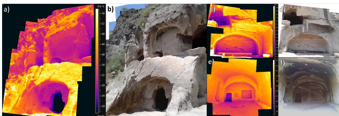
Figure 15. Close-ups of the criticalities in the cave systems acquired on S1: Mosaicked thermogram (a) and correspondent photo (b) of cave system characterized by persistent and spaced fracture system, mosaicked thermograms of intensively fractured cave system (c) with correspondent photo (d), mosaicked thermogram of single cave (e) and correspondent photo (f) characterized by spalling of the rock surface in the roof of the room, controlled by rock weathering and stress degradation.
