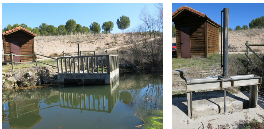
Figure 8.5: Hatch with manual opening for water diversion on Cega river.
