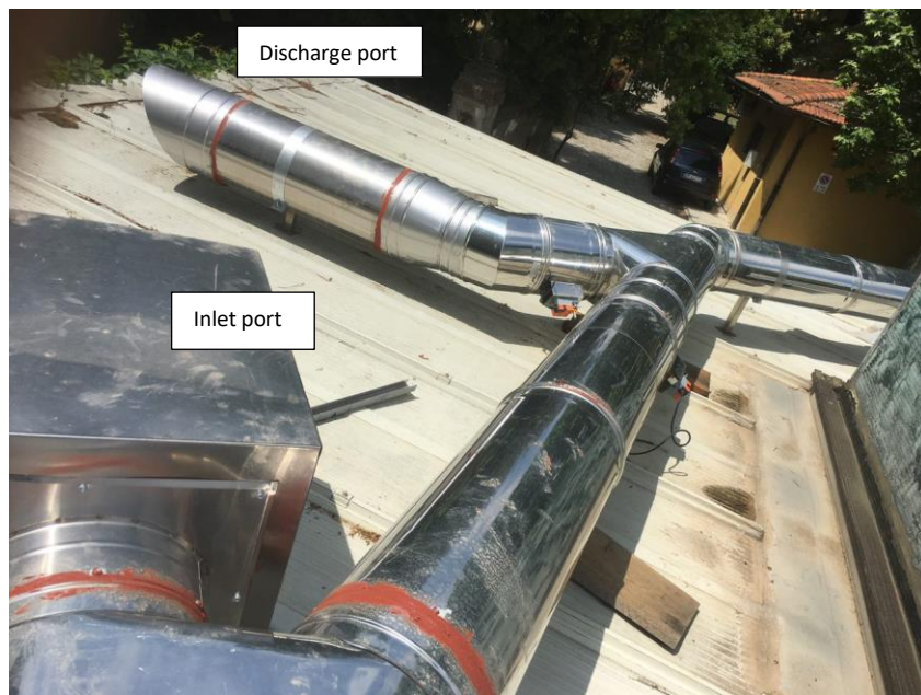
Figure 64, picture of the returning duct of the UniFi test rig
