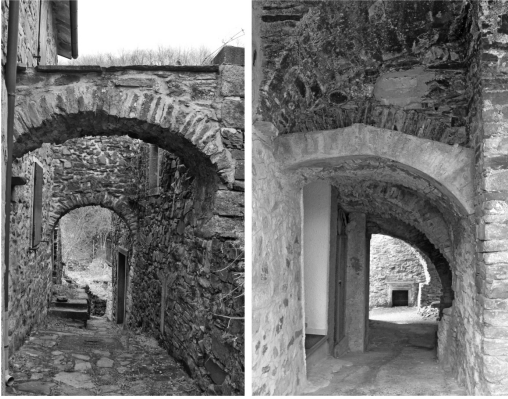
Figure 1. Traditional devices used to counteract horizontal forces in Lunigiana, Italy (L. Dipasquale).
