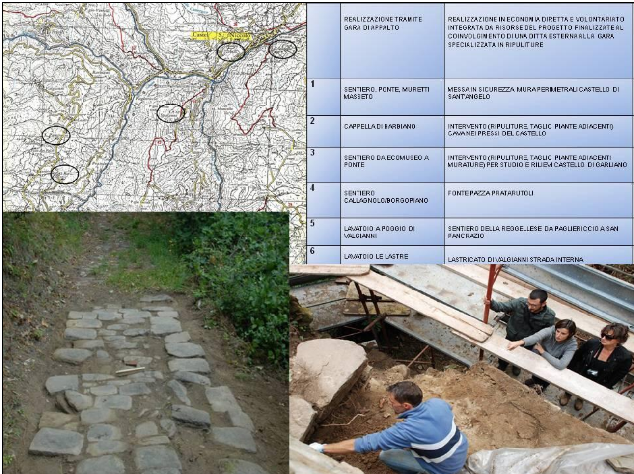
Fig. 25. 'Widespread worksites', for the recovery, restoration and enhancement of the territorially diffused heritage of tourist-cultural interest, carried out by small 'mixed' teams of specialists with the active participation of members of the local communities
