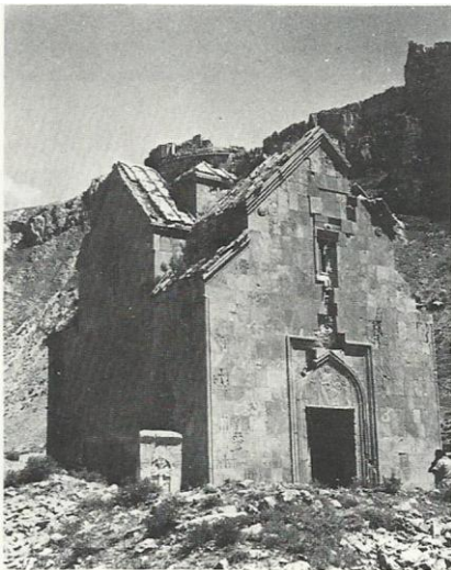
Fig. 35. Photo of the ruinous collapse of the drum and the cover cap.
