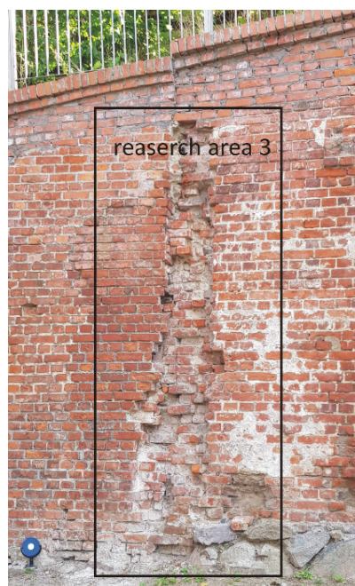
Figure 4. The research object 3, a damaged retaining brick wall.
