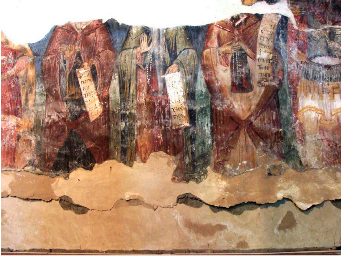
Figure I-5.3.11 Severe damage on the south wall of the church due to the rising damp. Key among these actions is repairing the hydraulic system in the southern part of the building, in order to make it fully operational 27 . The lack of maintenance caused vegetation to obstruct the canals, thus impeding them from carrying out their important function of containing and channelling toward the stream to the east of the church the great amount of water that flows down the slope. This water has also caused serious damage to the wall paintings on the southern wall of the church, especially before the restoration in 1999. Rising damp has brought about the swelling of the longitudinal timber elements present in the masonry, thus causing the detachment of plaster and consequently of the paintings 28 (Fig. I-5.3.11).
