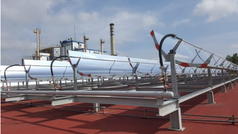
Figure 1.10: Application of parabolic trough collector in a dairy processing plant in Mexico [24].
