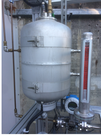
Figure 4.6: The expansion tank.
