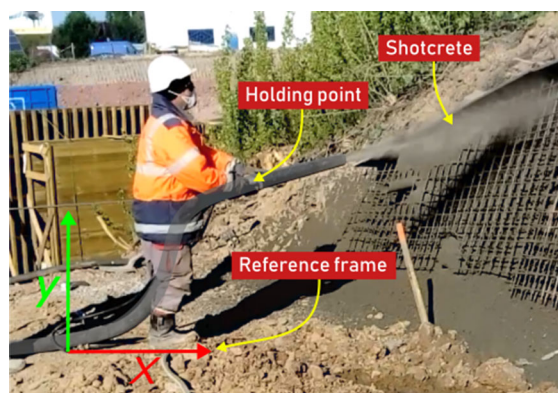
Fig. 2 A typical pose for the worker while holding the hose during a vertical-wall shotcrete projection
