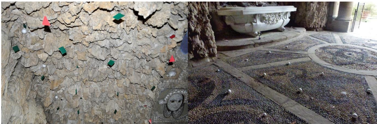
Figure 5. Pipes and nozzles highlighted with spheres and paper cuts on the vault and the floor.
