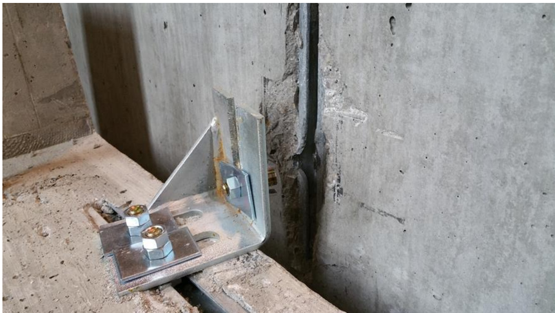
Figure 3-68: Test F17-01: the collapse of the anchor channel.
