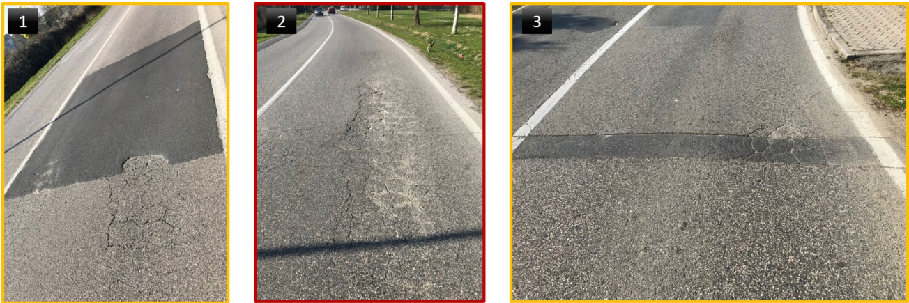
Fig. 12 Anomalies located in via Alessandro Scarlatti
