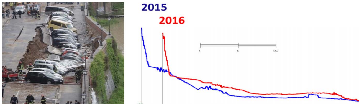
Figure 9. Documentation of wall failure occurred in 2016, and comparison of the update cross-section (in red, 2016) with the previous survey (in blue, 2015).
