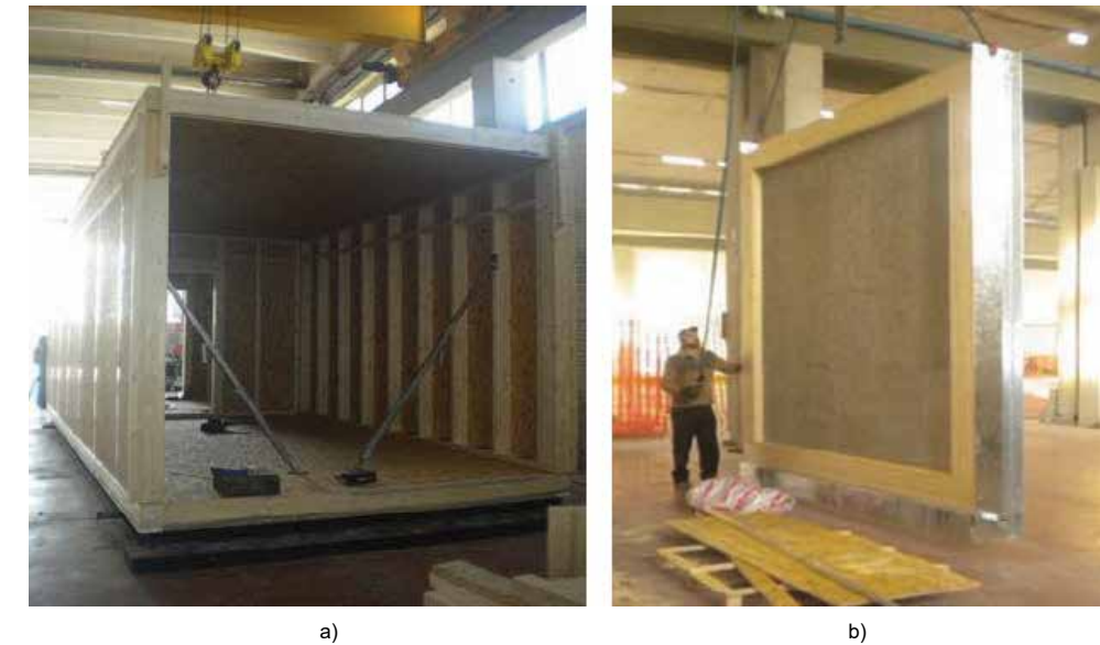
Fig. 1. a) The platform frame structure of Test Cell; b) The insulated removable wood façade for placing the test sample.
