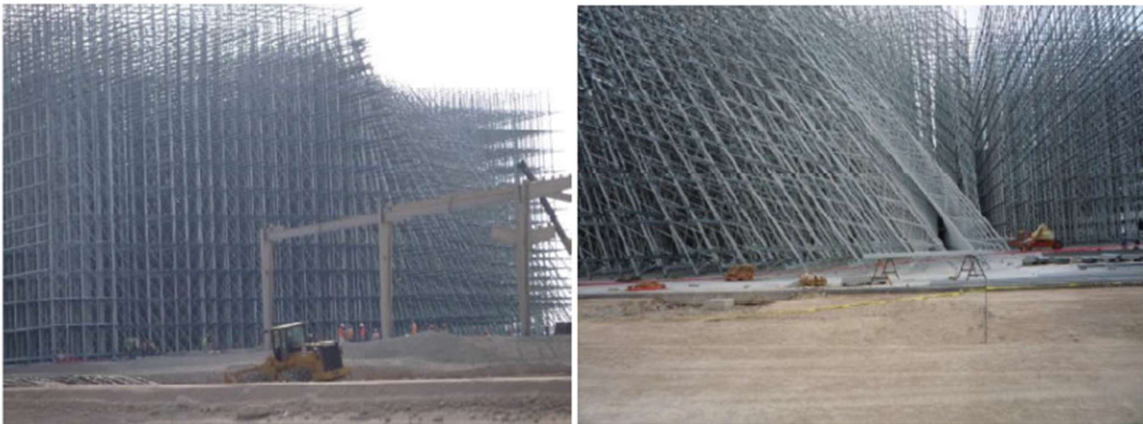
Figure 4-4: Partial collapse of an ARSW under construction.
