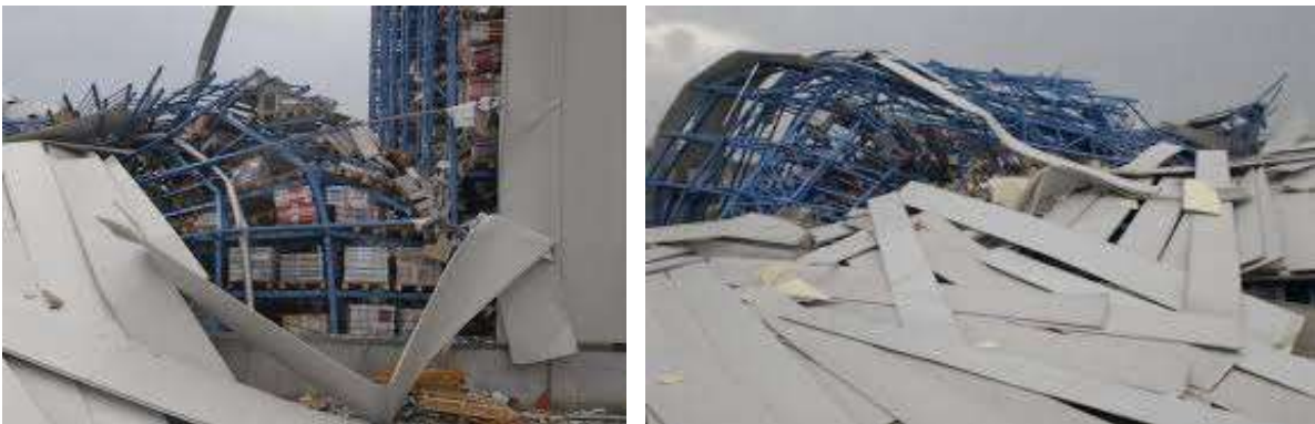
Figure 4-1: Collapse of Ceramiche Sant’Agostino warehouse after the “Emilia Romagna Earthquake” that happened in Italy in 2012.
