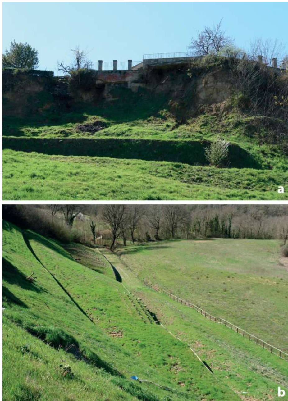
Figure 6 – Ricasoli village: a) compound slides which affect the N escarpment and b) slope stabilization works realized in 2013 (photos made on 20 March 2019).
