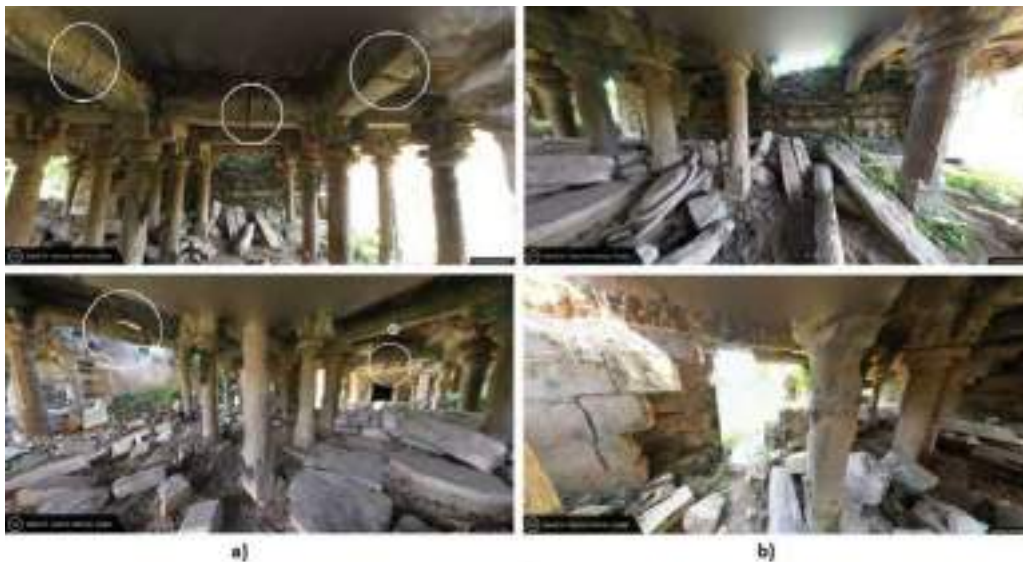
Fig. 8. VT environment that helps user identify (a) cracked beams (b) damaged walls.
