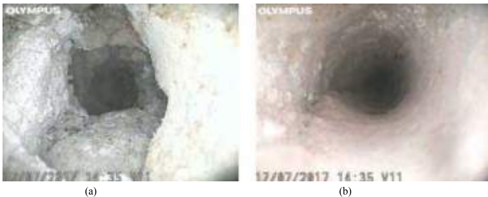
Fig. 8. Videoendoscopy V11 – from intrados: (a) View at 15 cm from the start of the drill, filling in unbound material; (b) Image at 5 cm from the start of the drill, brick and mortar elements.
