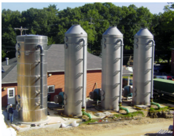
Example of packed columns in a \text{CO}_2 pre-stripping reactor Site Location: Natick, Massachusetts
