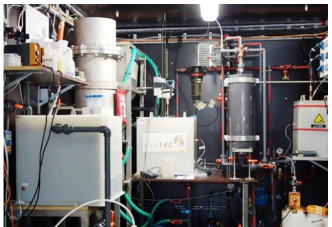
Container pilot plant by SUSTEC BV, THE NL Pilot of struvite precipitation in front of the stripping reactors
