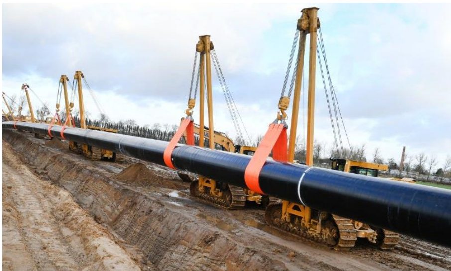
Figure 2.9: Image of a transportation pipeline.
