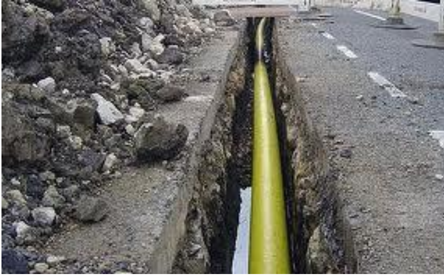
Figure 2.10: Image of a distribution duct.
