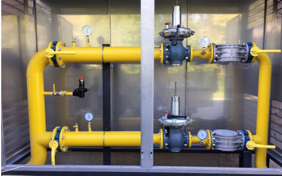
Figure 2.16: Image of a reducing station.
