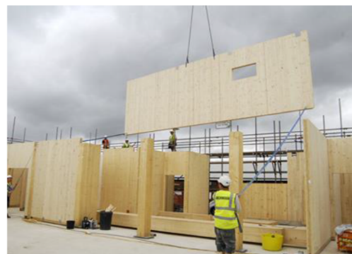
Image 03 - Panels can be transported on-site with a lower degree of prefabrication, i.e. structural wooden panels without external and internal finishes
