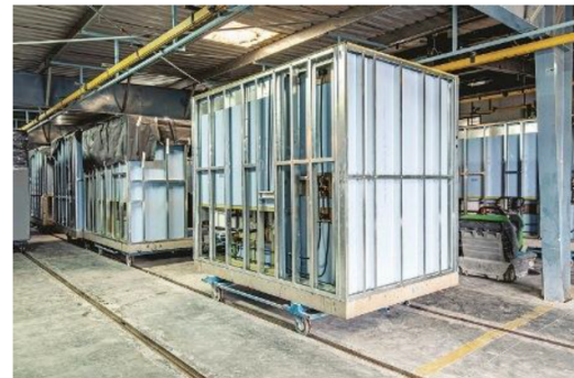
Image 03 – Steel modular units are also widely used for technical pods i.e. service cores usually employed for large-scale building complexes
