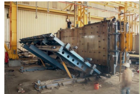
Image 02 – Manufacturing sequences: double mould for precast of sandwich panels, insulated with rigid polymer core
