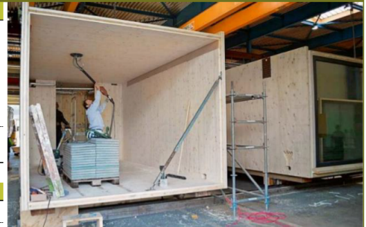
Image 01 – CLT modular units being assembled and integrated with cables and services inside a factory
