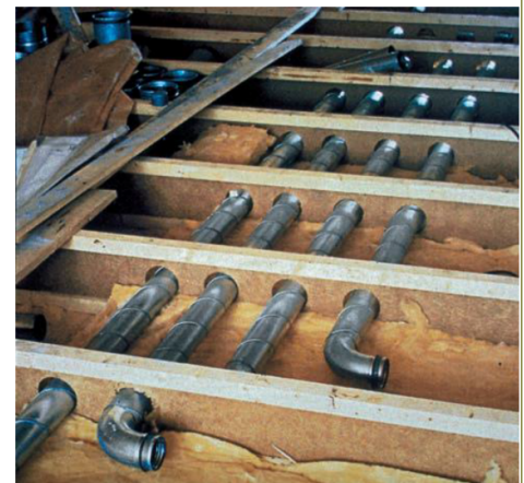
Image 02 – During manufacturing pipes and cables can be integrated providing holes in the panels in order to reduce on-site operations for services
