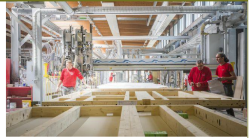
Image 01 – Sub-components and parts are assembled in panels following streamline sequences of industrial operations Credits: RubnerHaus
