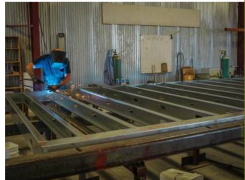
Image 01 – Cold Formed Steel profiles are off-site assembled by welding and mechanical fastening
