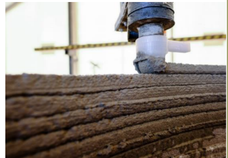
Image 03 – The binder can be constituted of different materials and mixtures; natural and eco-friendly resources as raw soil can also be used as part of the binder Credits: COBODO
