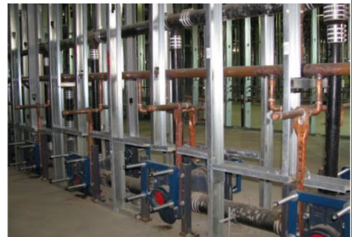
Image 02 – LSF panels offer the possibility for integrating technical services, optimizing internal space distribution
