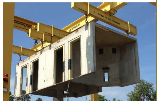
Image 03 – Modular units installed on-site: due to dimensional restrictions, space layouts and flexibility are reduced
