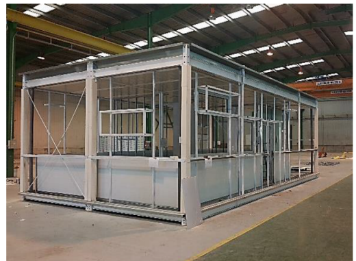
Image 02 – Portable modular units assembled inside the controlled environment of the factory. The picture shows the steel skeletal structure infilled with steel sandwich panels
