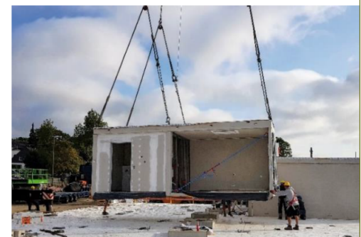
Image 02 – Installation phases of modular units on site. Volumes come with a lower degree of completion and need further on-site operations to be finished Credits: Solid Box
