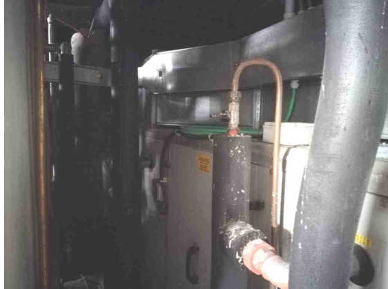
Fig. 7. Room 41: AHU in the attic room.
