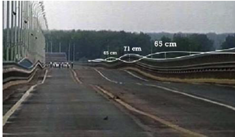
Figure 1.3. Views of the Volgograd bridge (top) and of its deck during the VIV phenomenon observed in 2010 (bottom) (Corriols and Morgenthal, 2012).
