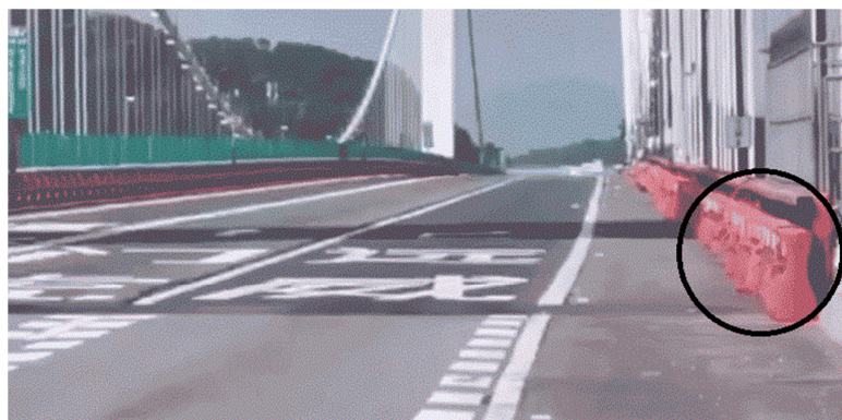
Figure 1.4. View of the structure (top) and of the deck (bottom) of the Humen Bridge. In the deck view, the lateral walls applied temporarily are indicated.
