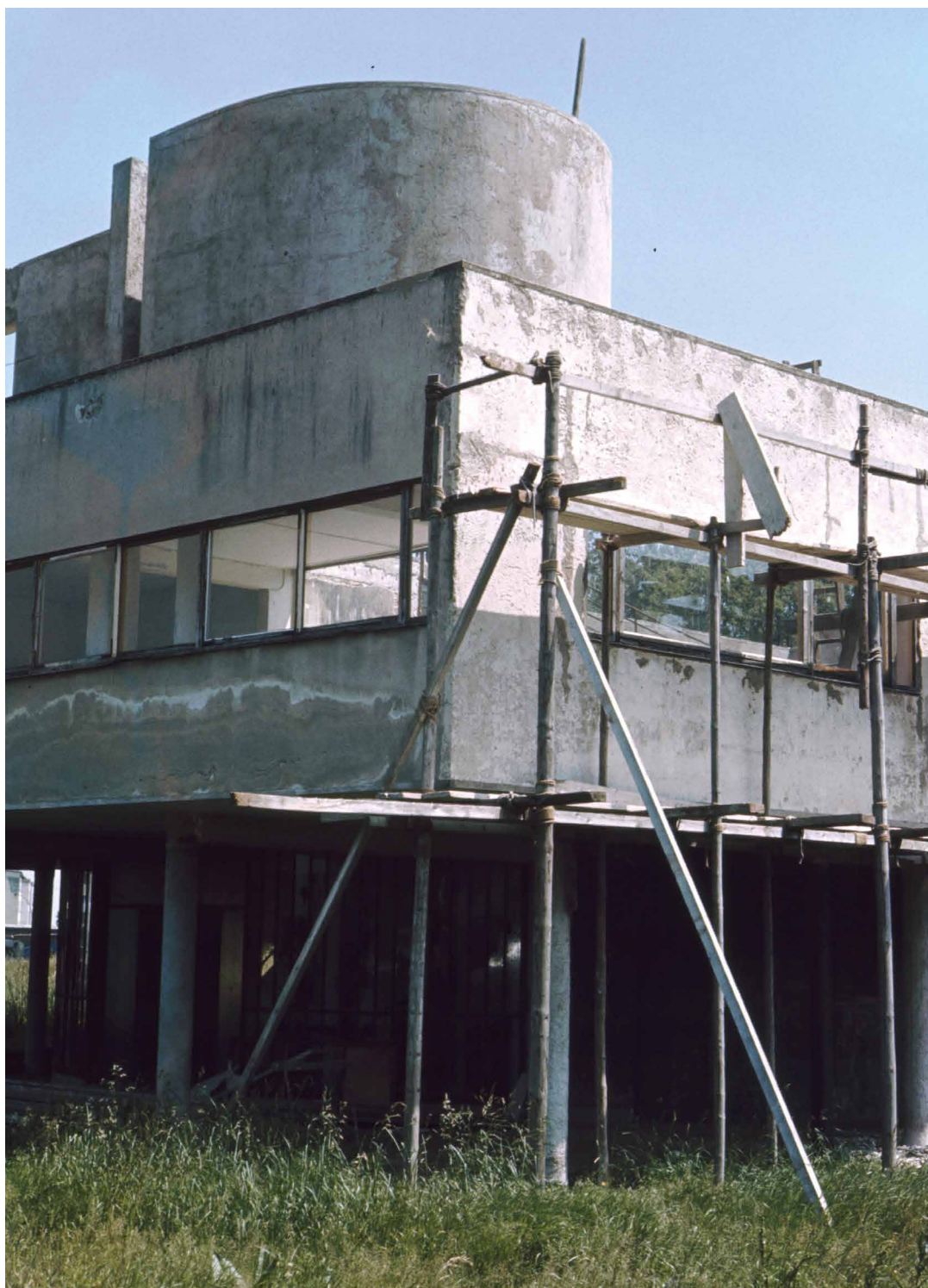
FIG. 2 Villa Savoye, Scaffoldings during restoration works, 1966 (picture by Félix Thyès). FLC – Fondation Le Corbusier, Paris.
