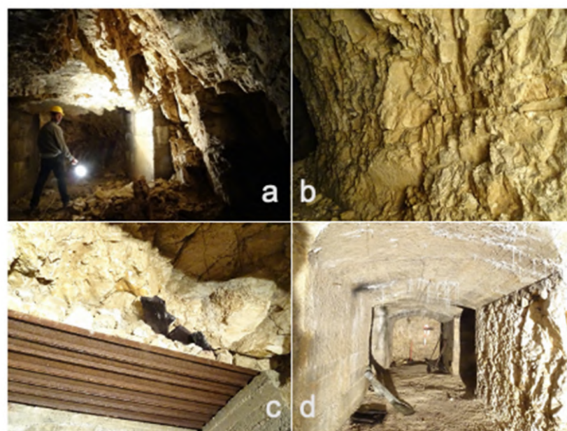
Figure 2. View of (a) vault collapse within the tunnel; (b) limestone outcrop; (c) vault protected by metal liner; (d) limestone outcrop + concrete coating.
