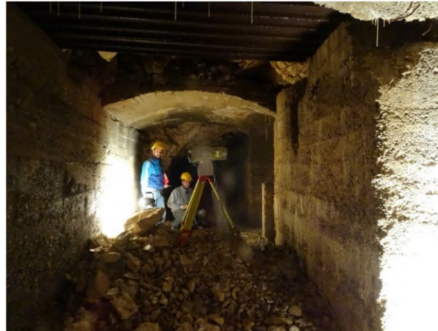
Figure 4. Laser scanner working in correspondence of a vault collapse.
