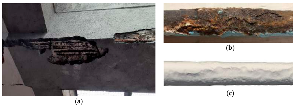
Figure 11. RC beam from the car park after concrete cover removal (a); details of the bar as extracted (b) and by tomographic scan (c).
