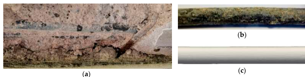
Figure 9. RC beam of the external colonnade after concrete cover removal (a); details of the bar as extracted (b) and by tomographic scan (c).
