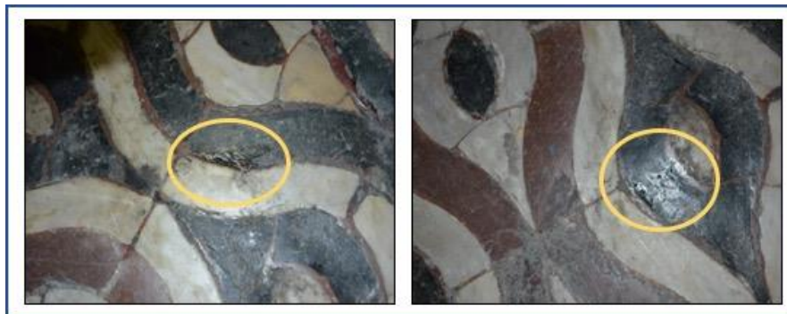
Figure 7. Detail of the baptistery pavement showing the water rising from the subsoil (yellow circles).
