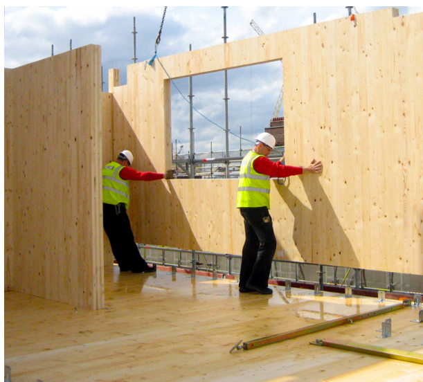
Fig.45 - Sistema costruttivo a parete massiccia in legno (Cross Laminated Timber, CLT) (Credits: Simpson Strong-Tie: www.strongtie.co.uk )
