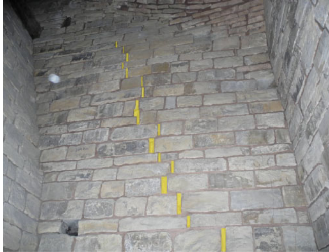
Figure 4. Transversal partition wall above the scarsella; the crack (in yellow) sealed by vertical plates is visible; the extrados of the dome can be seen on the left.
