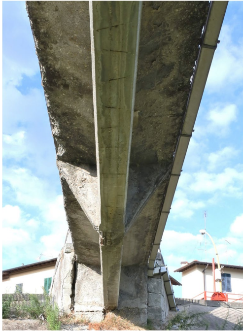
Fig. 7 Walkway, diffuse concrete corrosion
