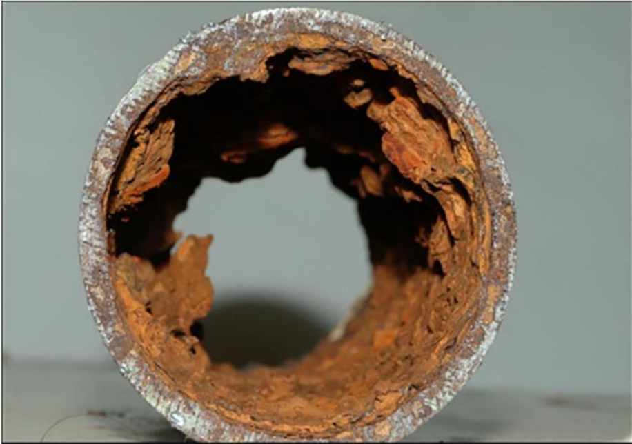
Figure 18 Effects of microbiologically induced corrosion in stainless steel pipe carrying chlorinated potable city water
