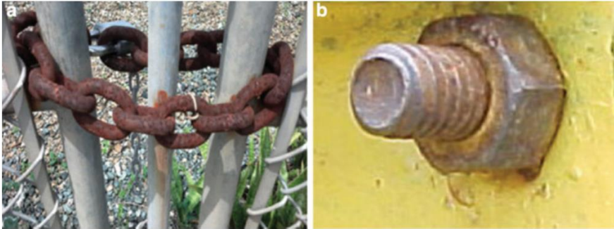
Figure 16 Galvanic corrosion of a (a) steel alloy chain and (b) carbon steel bolt-nut coupling
