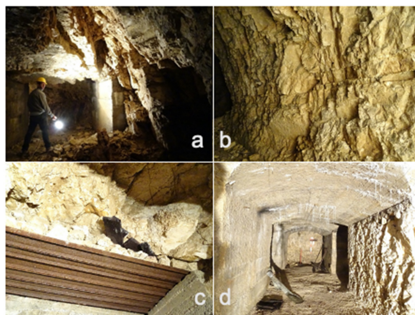
Figure 2. View of (a) vault collapse within the tunnel; (b) limestone outcrop; (c) vault protected by metal liner; (d) limestone outcrop + concrete coating.
