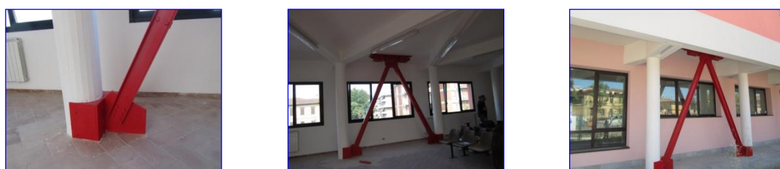
Fig. 20. Detail and general views of the other DB alignment parallel to x in the pilotis wing.
