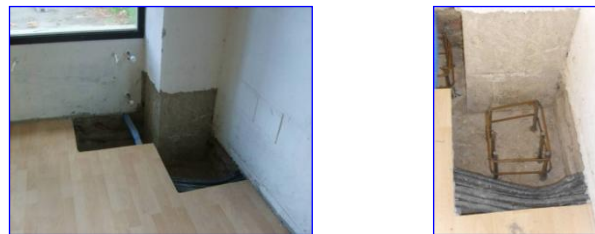
Fig. 18. Preparation of the anchorage zones of braces to the foot of a column.
